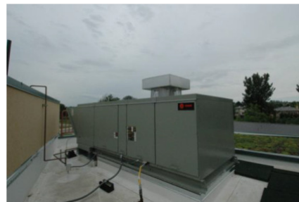
High Efficiency HVAC
